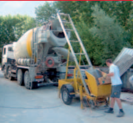
Einfache Stahlfaserzugabe in den Fahrmischer. Steel fibres can be easily added to the cement mixer.
