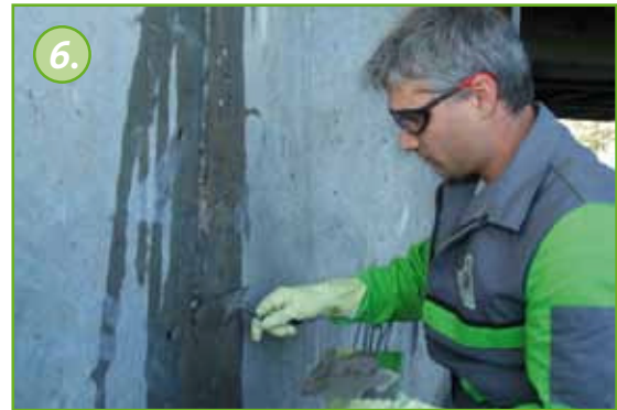
Close the crack along its course with KÖSTER KB Fix 5. Closing the crack prevents injection material from prematurely flowing out of the crack during the injection. Setting time is approx. 5 minutes, depending on the surrounding temperature and humidity.
